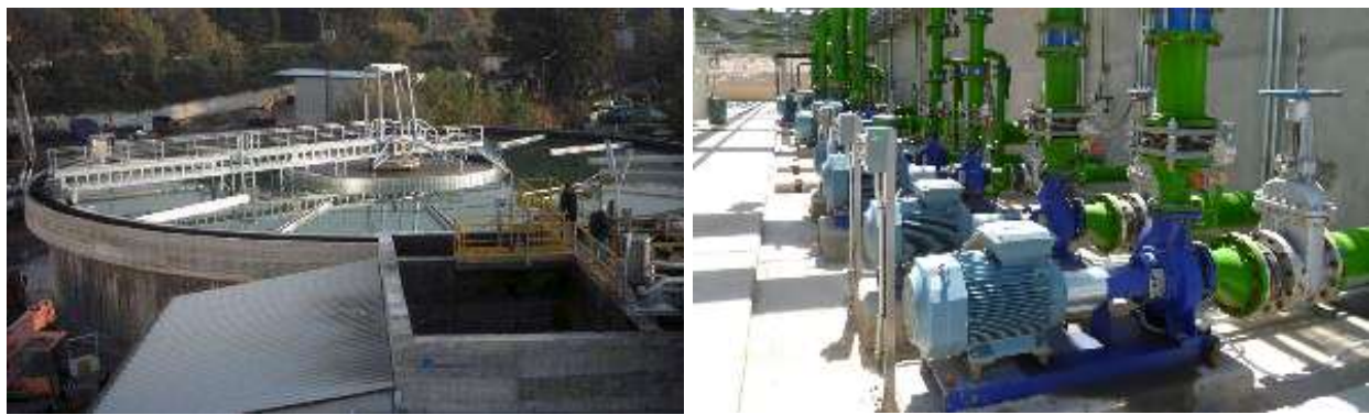
Figure 1.6-4.: photos of a circular decanter and a pumping station in a Water Treatment Plant [3]
