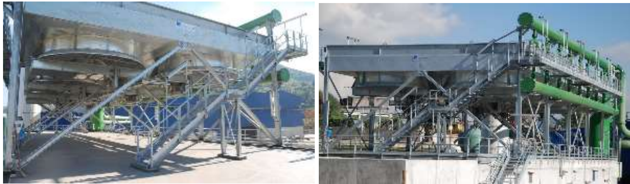
Figure 1.6-3.: Photos of air coolers, the alternative to evaporation towers, used to avoid water loss from evaporation [3]
