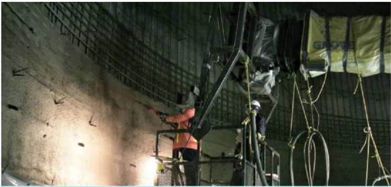
Figure 10.3-4.: Shotcrete applied atop reinforcing steel forming the strong shell of the dome silo [1]
